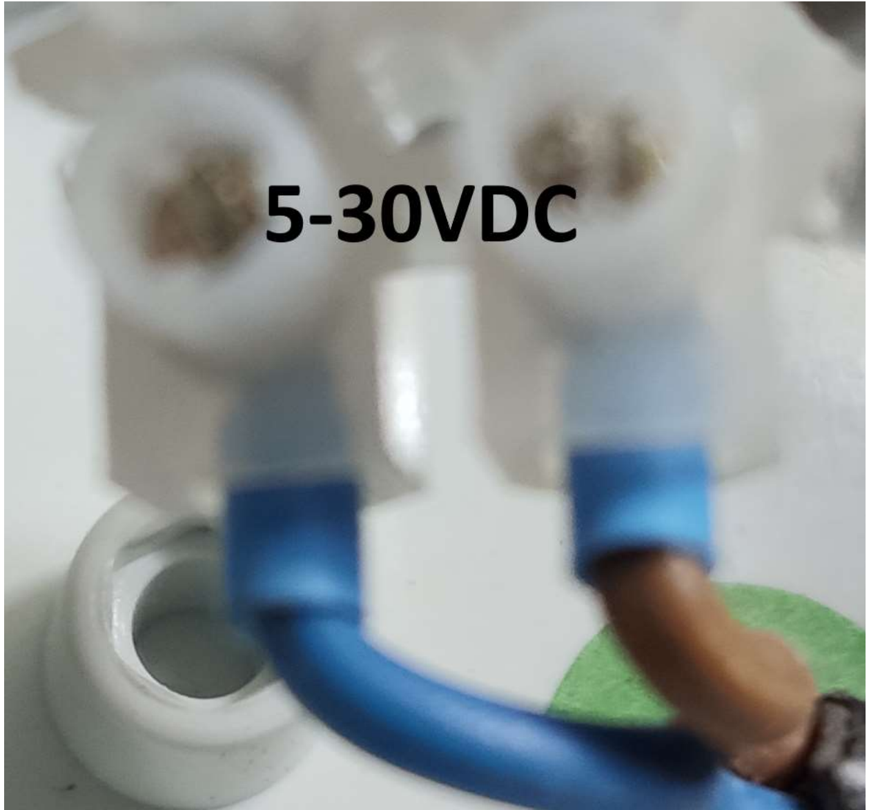
Inside white box on side of Z axis wiring to spindle
